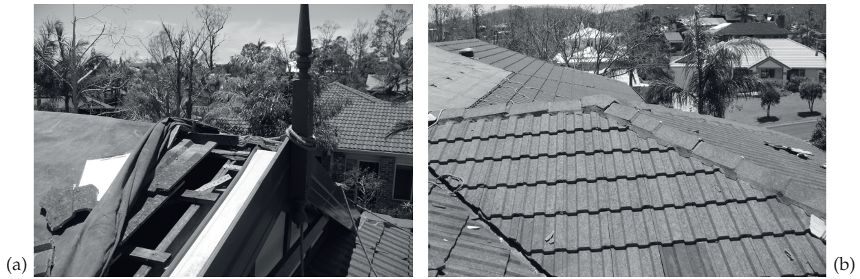
Figure 12: Details of ridge tile roof failure and hip tiles without mechanical fastening – (a) view of failed ridge tiles under tarpaulin; and (b) view of ridge and hip tiles, which are still in place but some without mechanical fasteners.
