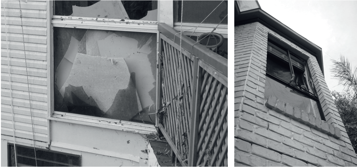
Figure 14: Typical wind-borne debris damage to windows.
