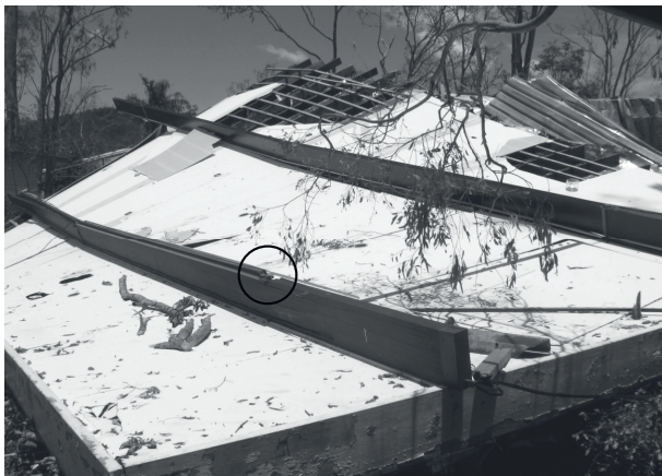
Figure 17: General view of upside-down roof.
