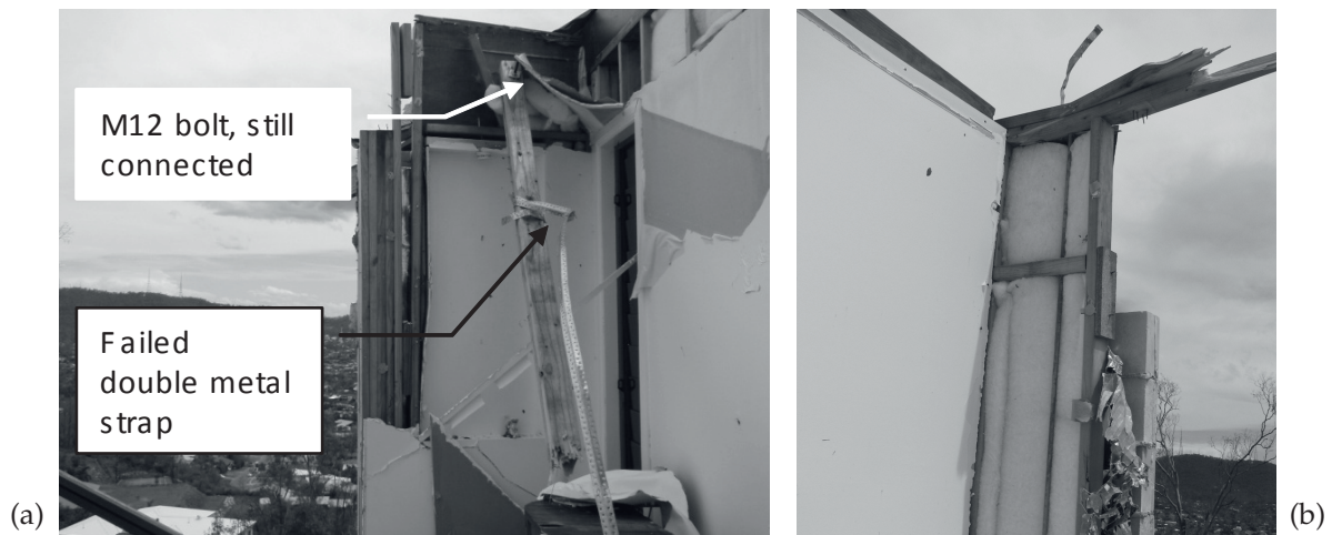
Figure 22: Lintel hold-down, combination of metal straps and HD bolts at far end of ply bracing frame – (a) one end of top plate, strap failed and M12 bolt too far away; and (b) M16 bolt too far from lintel and not configured as per AS1684.
