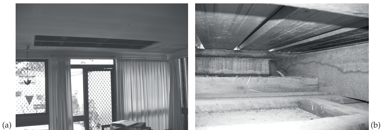
Figure 11: Overflow of gutter water into ceiling space – (a) view of hole in ceiling, after collapse of one plasterboard panel; and (b) view inside ceiling space showing water staining on rafter overhang.
