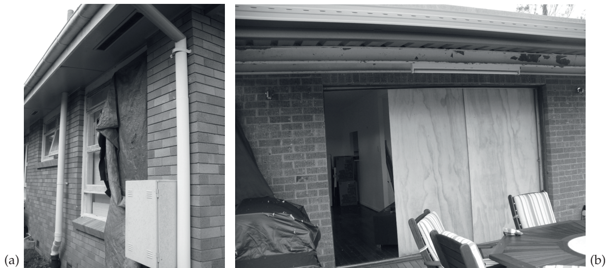
Figure 13: Typical windows and doors failure – (a) hail damage and window pushed in; and (b) sliding door failed.
