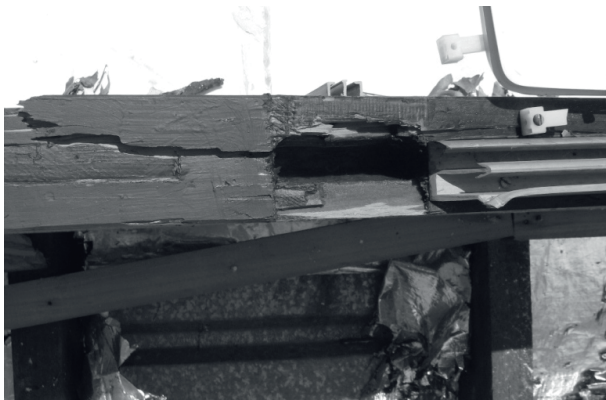
Figure 18: Typical view of a failed mortice joint to roof beam.
