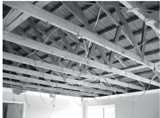
Figure 8: General view of typical ceiling collapse (unsarked tile roof).
