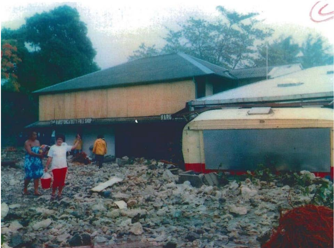
Typical damage from overtopping flows and rubble
