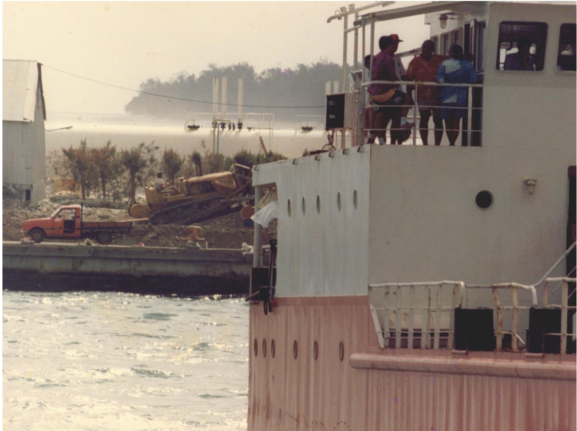
Shot after cyclone of Avatiu harbour showing a dozer clearing away rubble buildup
