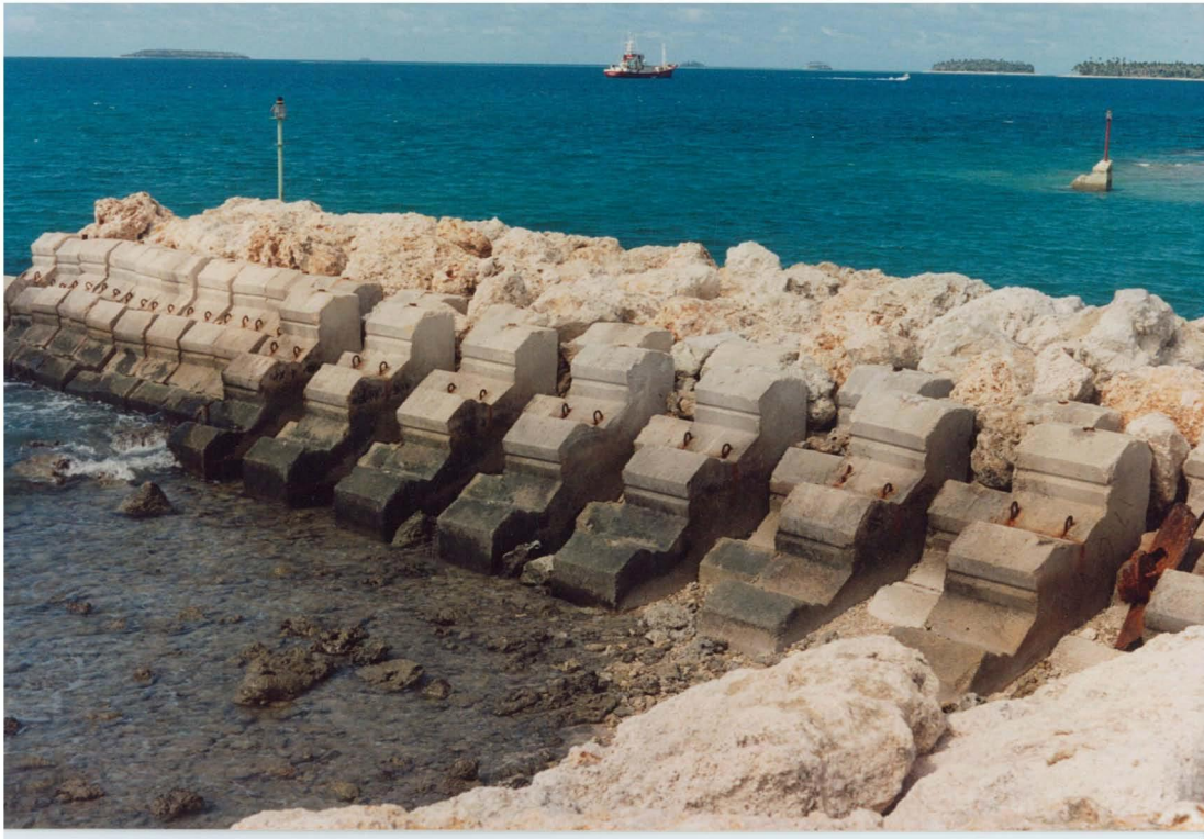
West Entrance Breakwater, Touliki Harbour, Nuku'alofa, Tonga, showing front profile of 'Eua Blocks (Tip constructed on rubble foundation replacing weak substrate)
