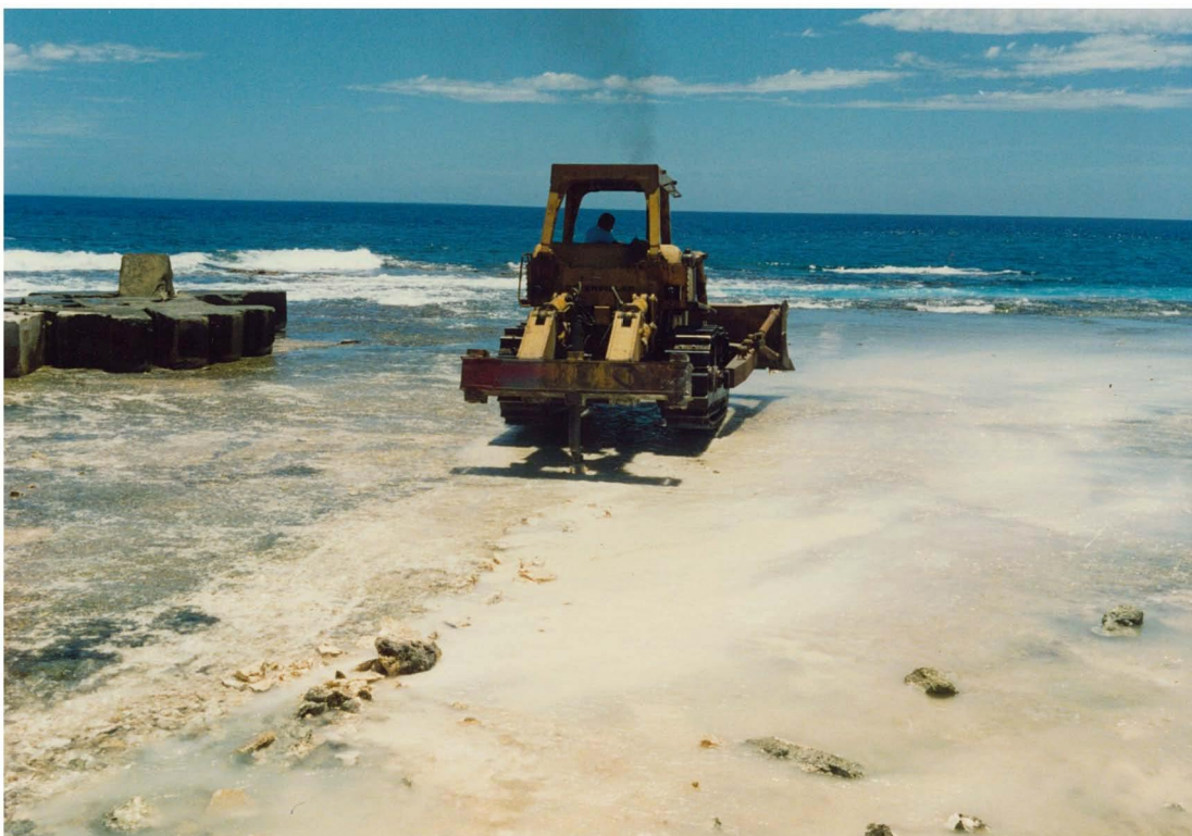
Dozer ripping cemented reef flat in preparation for placing concrete blocks, South Breakwater, Nafanua Harbour, 'Eua
