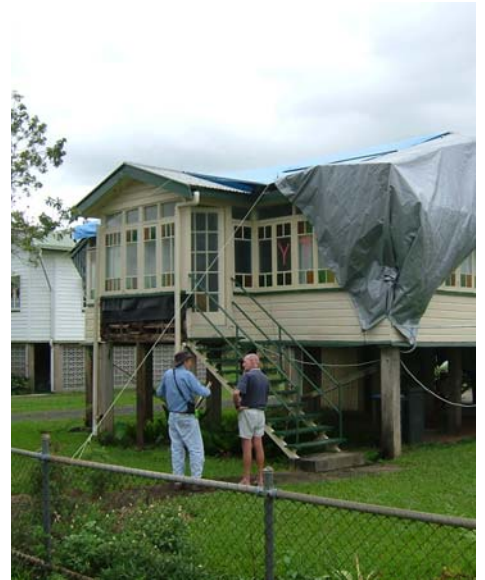
Above: JCU Cyclone Testing Station Senior Research Engineer Campbell Leitch discusses the roof damage to an Innisfail house with the owner. On behalf of Willis Re, SEA and the JCU-CTS undertook a detailed inspection of damaged homes in early May, correlating the damage with assessed insurance losses.
