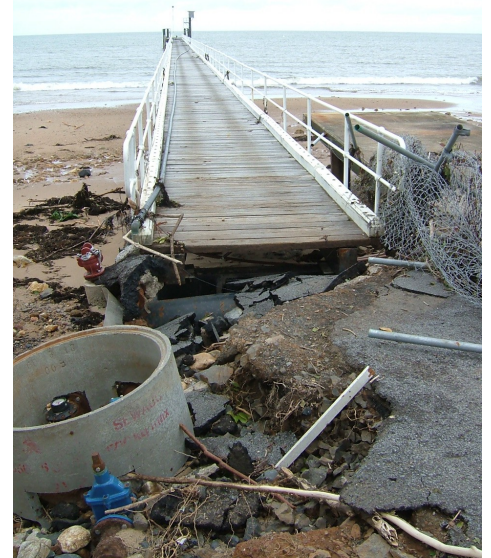
Above: Clump Point jetty after TC Larry in 2006 produced peak stillwater levels more than 2 m above the high tide levels between Cardwell and Cairns.
